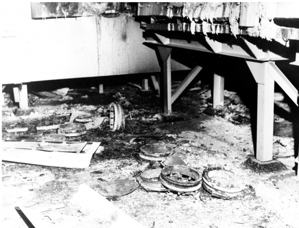
Figure 4.6: A glovebox area in Building 776, totally destroyed in the May 11, 1969, fire, the most expensive industrial fire to date in U.S. history, costing close to $50 million, not including the one metric ton (2,240 lbs.) of plutonium burned in the fire.
